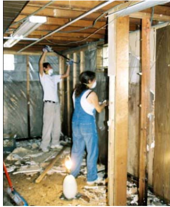
Peter and Sandy Kurowski gut the wall in the basement of a home in East Chicago.
