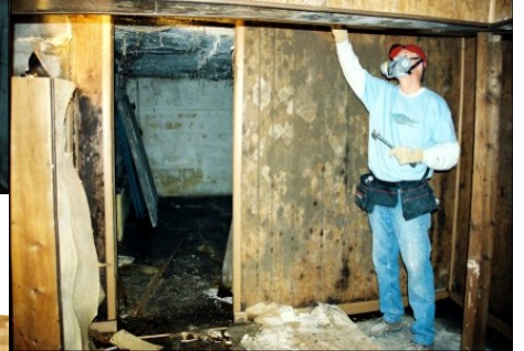
Tom Retseck works with team to tear out paneling covered with mold.
