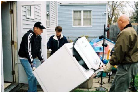
Jeff and Donna Smolinski and Walter Krantz haul appliances out of Wihemena's home in Gary prior to gutting and sanitizing.
