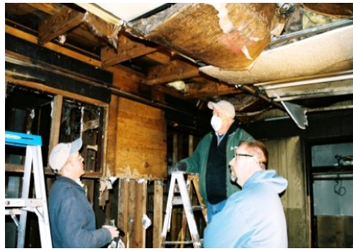
Kevin Grooms, Bob Rinearson and Keith Burke assessed the plan to rebuild the load bearing wall.
