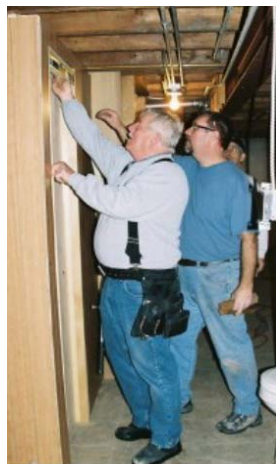
Bob Rinearson and Keith Burke, St. Joseph the Carpenter Ministry Coordinator, use a level before securing the door for Barbara's bathroom.
