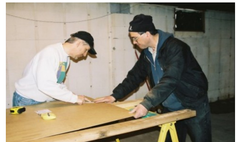
Joe Melko and Dave Leydet measure plywood before cutting it to rebuild Barbara's basement bathroom.
