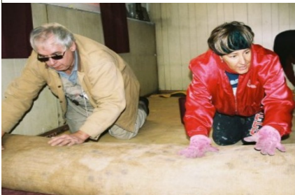
Terry Willie, the newest member of Faith Without Borders and resident of Winfield, works with Jenny Krol to roll up flood stained carpeting
