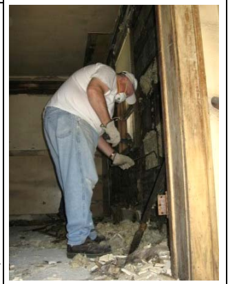
Dan Majchrowicz pries away plaster down to the studs to gut the home.
