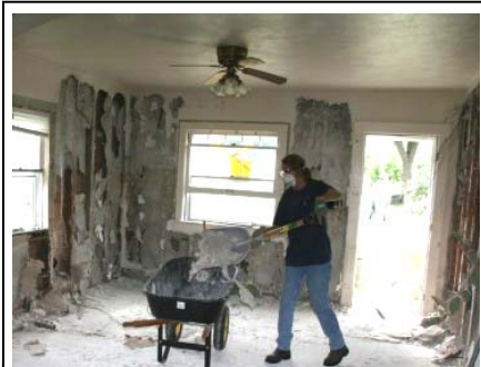
Barb Popiela shovels debris from Betty's living room into a wheel barrel.
